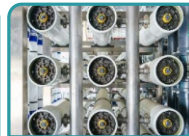
RO Membrane Treatment
